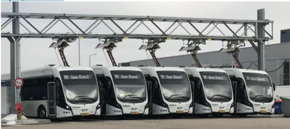
Figure 10 450kW opportunity chargers at the Schiphol airport
